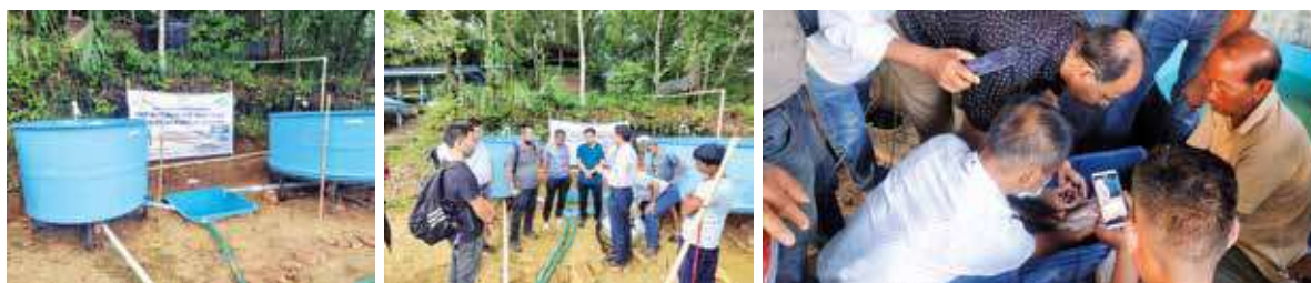
Installation of FRP hatchery for Demonstration of Mass Scale Seed Production in Mizoram and Manipur
